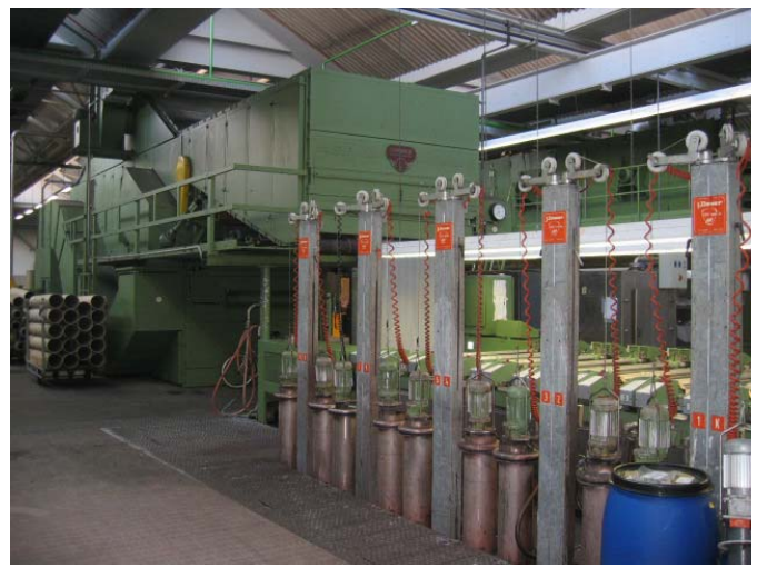
with 3 sections gas heated dryer
