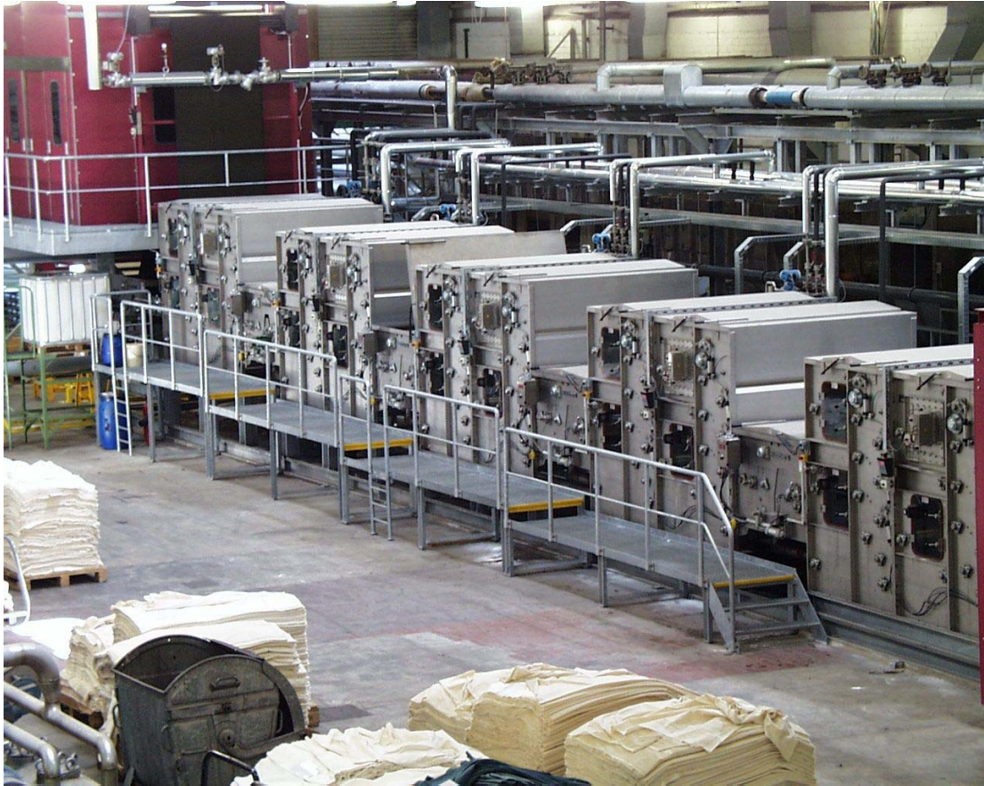
6 wash boxes, type pile flush – the newest type of Kuesters–low water consumption
