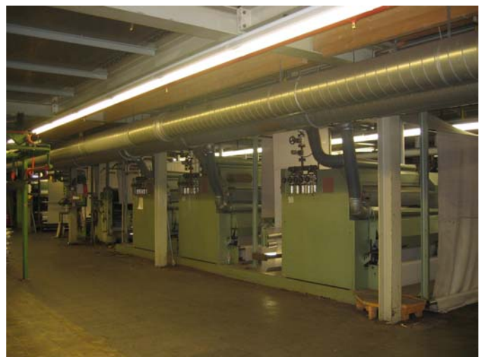
Finishing line for velours
