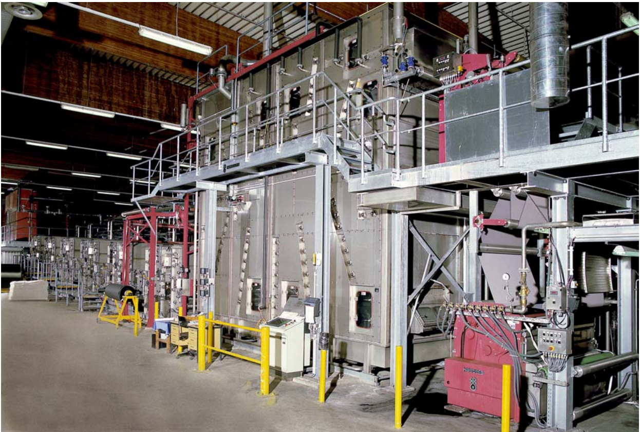
Continuous dyeing range Kuesters , installed end of 1999 , started in 2000
