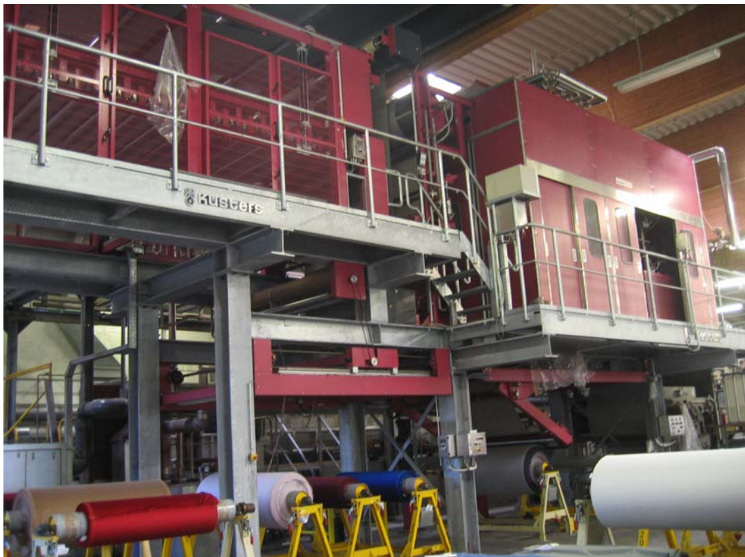
6 drums Wumag drum dryer , accumulator and two batching arms for non stop processing
